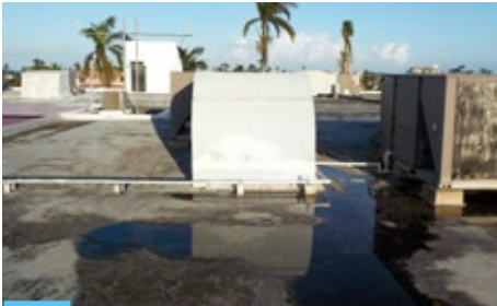
Before the implementation of Daikin's VRV solution.
