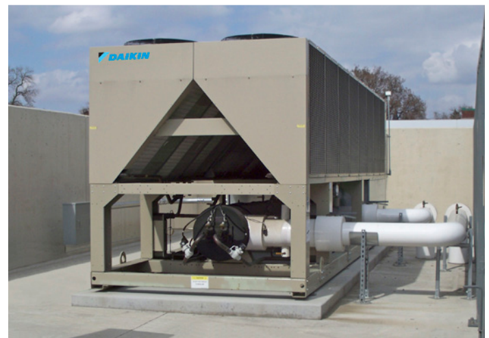
The 210-ton Daikin Pathfinder Chiller installed at Whittier Clinic contributed to LEED points in two areas of sustainability – optimized system efficiency (EAc1) and enhanced refrigerant management (EAc4).
