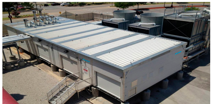
The plant and cooling towers accommodate capacities for Phase 1 and 2 of construction, with additional capacities slated for 2017 and 2019.
