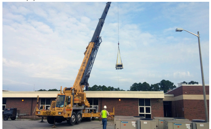
21 Daikin Rebel VAV, single-zone units provided the indoor air quality and energy saving solutions the district required.
